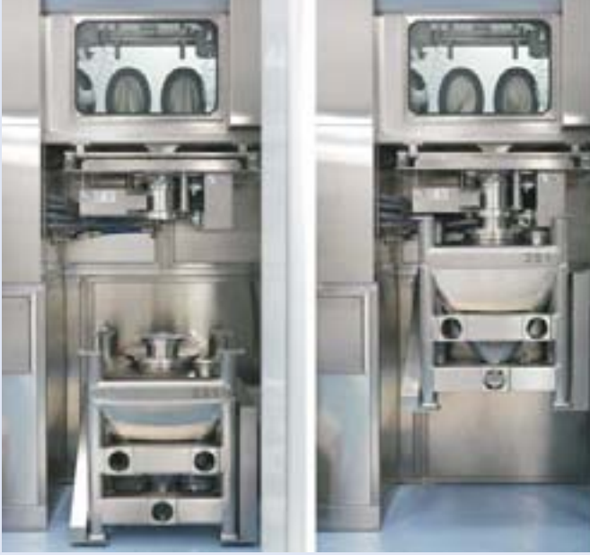
Product transfer to the PH-Bin by using TwinValve
