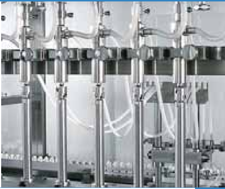
CIP System on filling pumps
